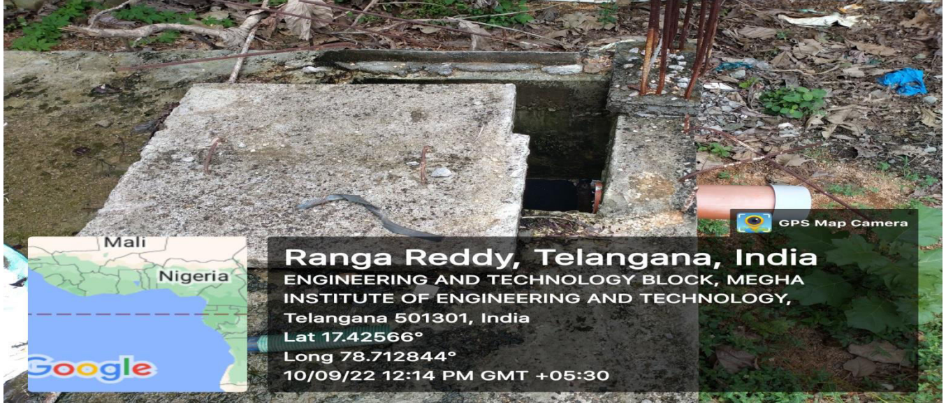
Water water collecting Tank.
